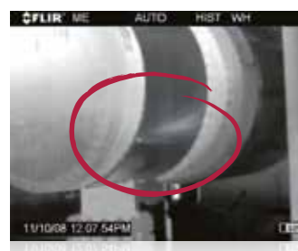
Gas leak in a petrochemical plant
